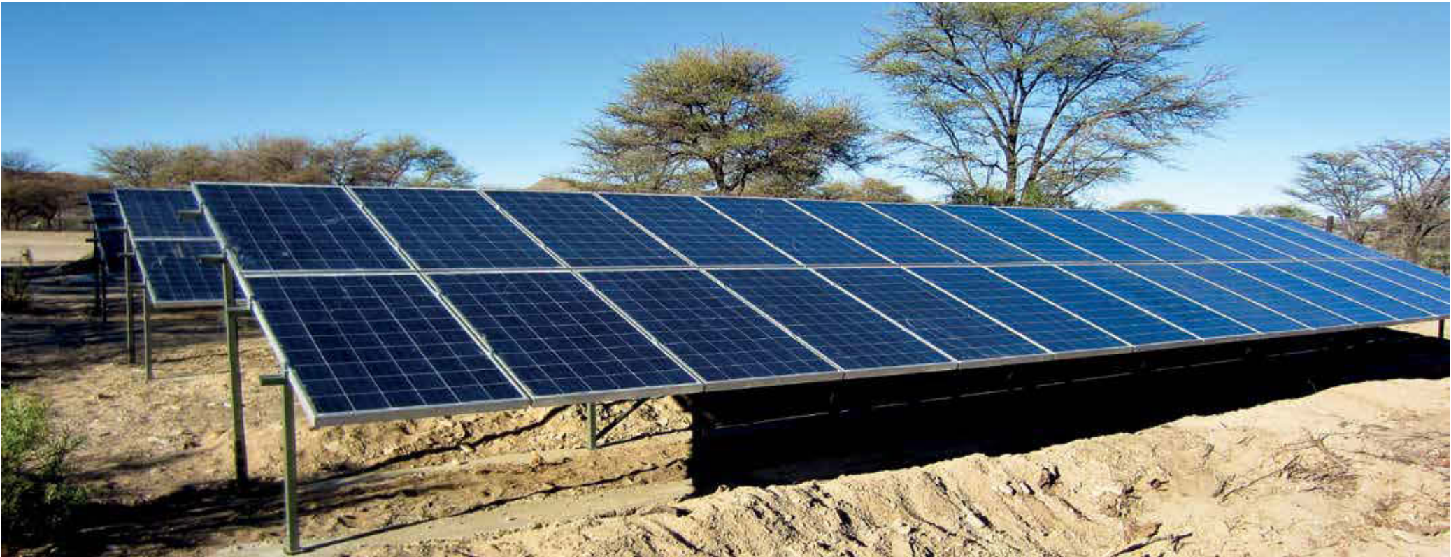
Solar panels at Neuras Winery, Namibia.
