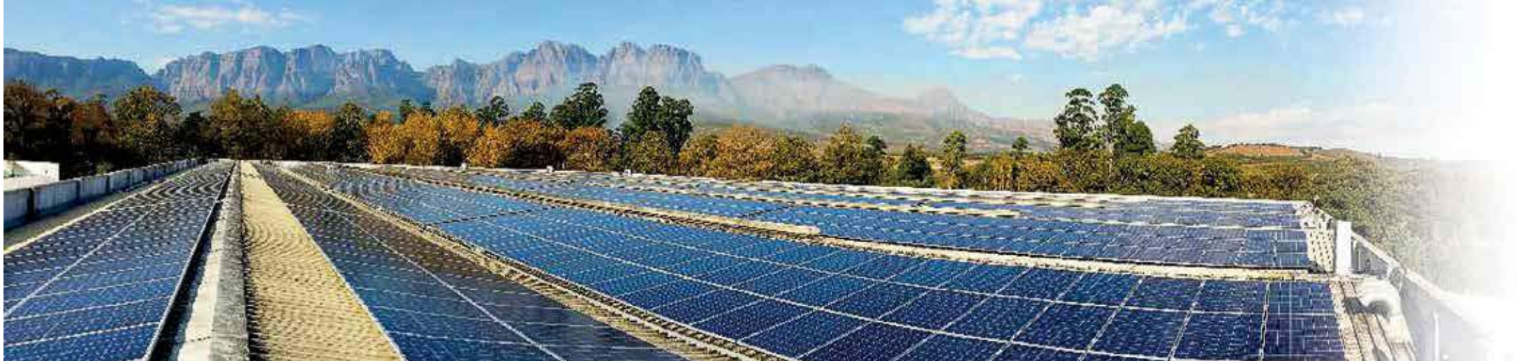
Lourensford PV (photovoltaic) installation.
